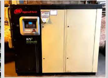
INGERSOLL RAND R75N AIR COMPRESSOR
