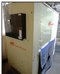
INGERSOLL RAND REFRIGERATED AIR DRYER
