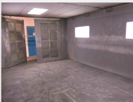
COMPLETE PAINT BOOTH
