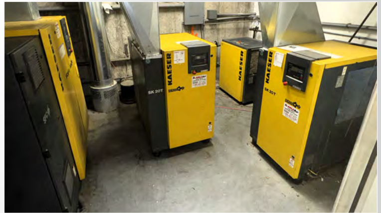
VIEW OF AIR COMPRESSORS
