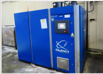
QUINCY QGV-100 100HP ROTARY SCREW TYPE AIR COMPRESSOR
