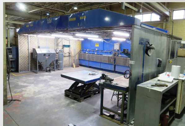
FILTER 1 DUSTRON DEBURRER & GRIND DUST FILTRATION BOOTH
